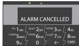
ALARM CANCELLED Keypad Display
